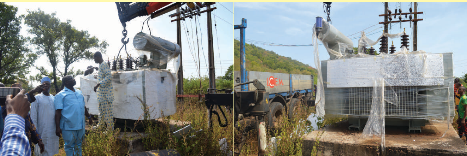
Donation of Sub Station Transformer to Oke-Ode Community, Ifelodun Local Government of Kwara State
