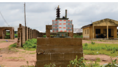
Donation of Transformer
