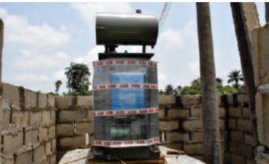
Donation of Transformer
