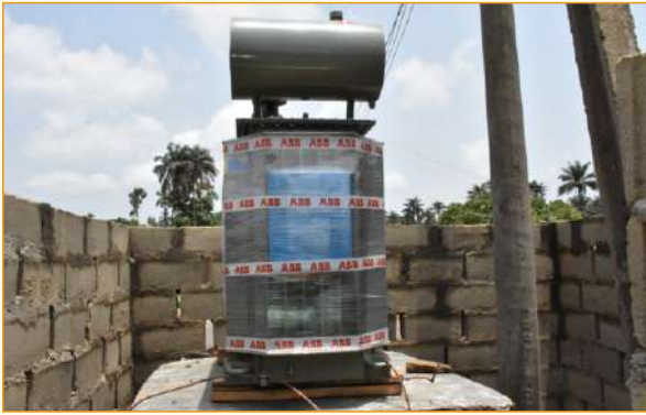
Side view of the transformer
