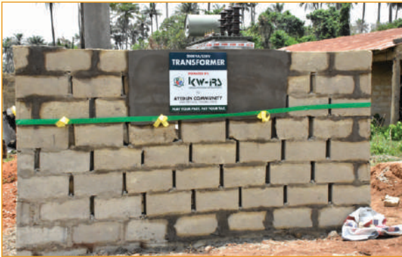
Front view of the installed transformer in Ayedun
