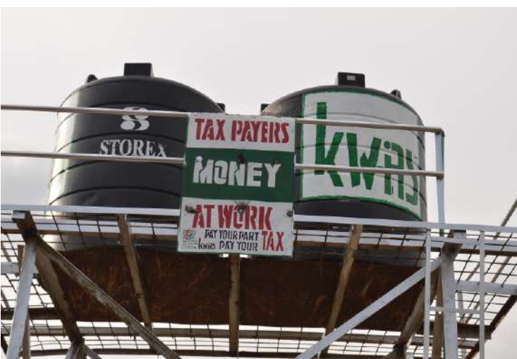
Provision of Overhead Tank for Water storage
