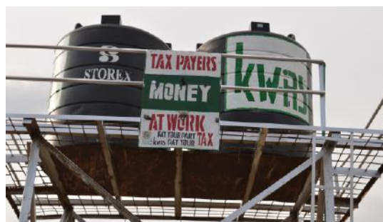
Borehole and overhead Tank at Alapa Market
