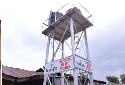
Borehole and Overhead Tank at Oke Ose Kara Market
